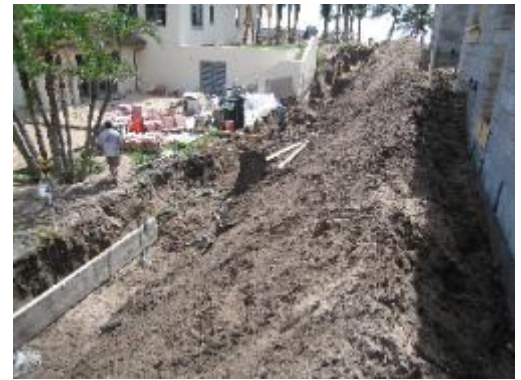
Excavated area is filled. More fill is brought in to next elevation.
