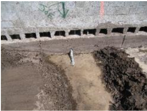
Footer for wall excavated. Auger cast Piles were used for wall support. Wall Construction begins. Helical piles Installed in lower section for lateral wall Support.
